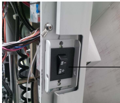
Main power switch (Public Canada)
